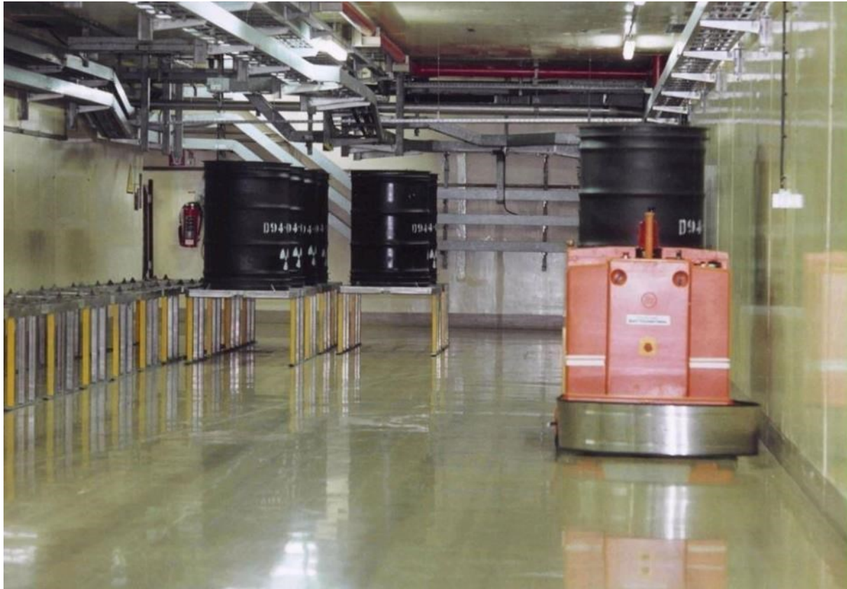
Figure 29: The WAB building (empty drums waiting for the next conditioning campaign)
